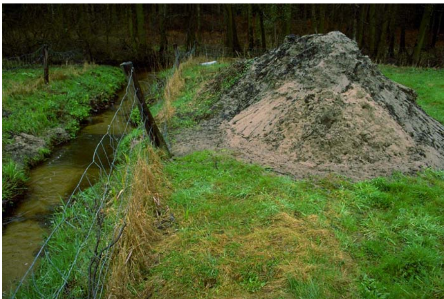
Fig. 2: Sediment trap in the Endeholz Ditch just before the confluence with the Lutter river (background) with the mound of sandy and organic material which was taken out of the trap from 1991 to 03. April 1998. The size of the mound shows the large amount of material carried by this small ditch.
